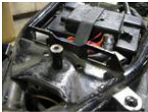
Use a cut-off wheel and grind off the upright "gate" which was the mount for the front of the stock Special seat.
